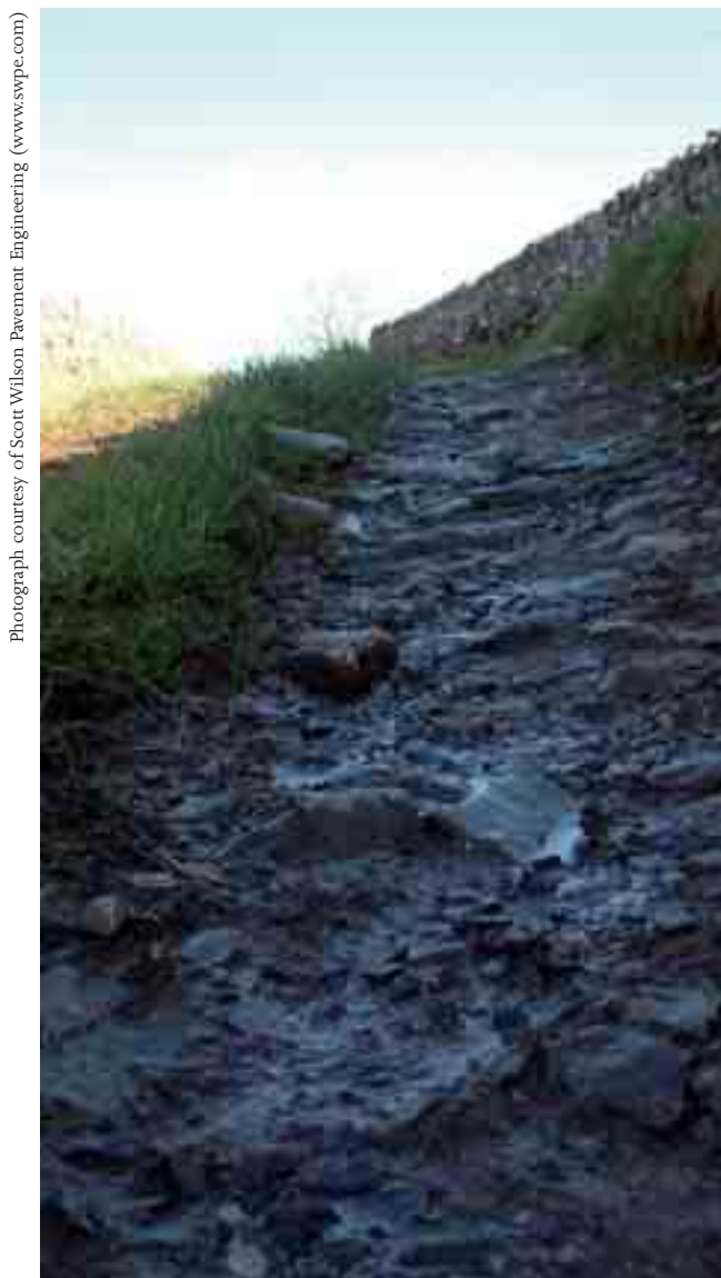
Surface erosion of a route on a gradient
